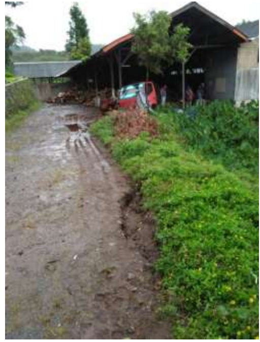
Ground cracking in tea factory - Nirmala.
