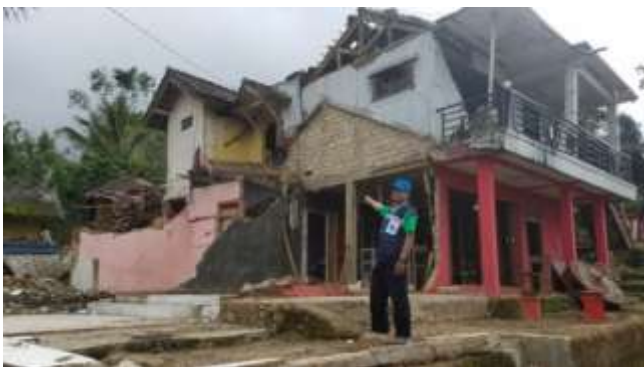
House damage totally at Citalahab
