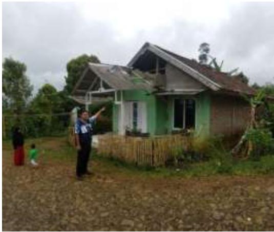
House damage slightly in Sinarsari
