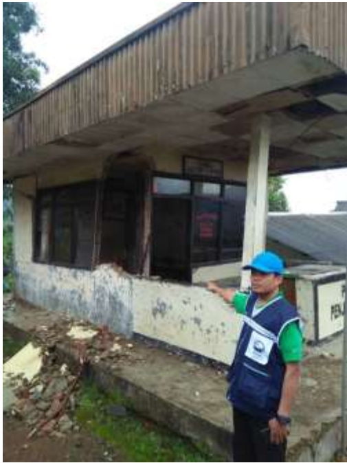
Building Security damage at Nirmala.
