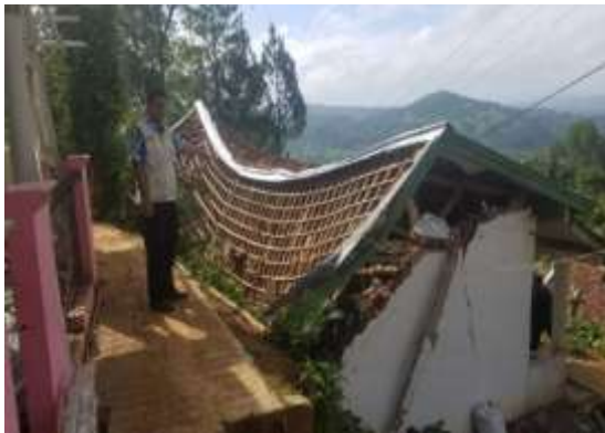
House damage totally in Bantarsari
